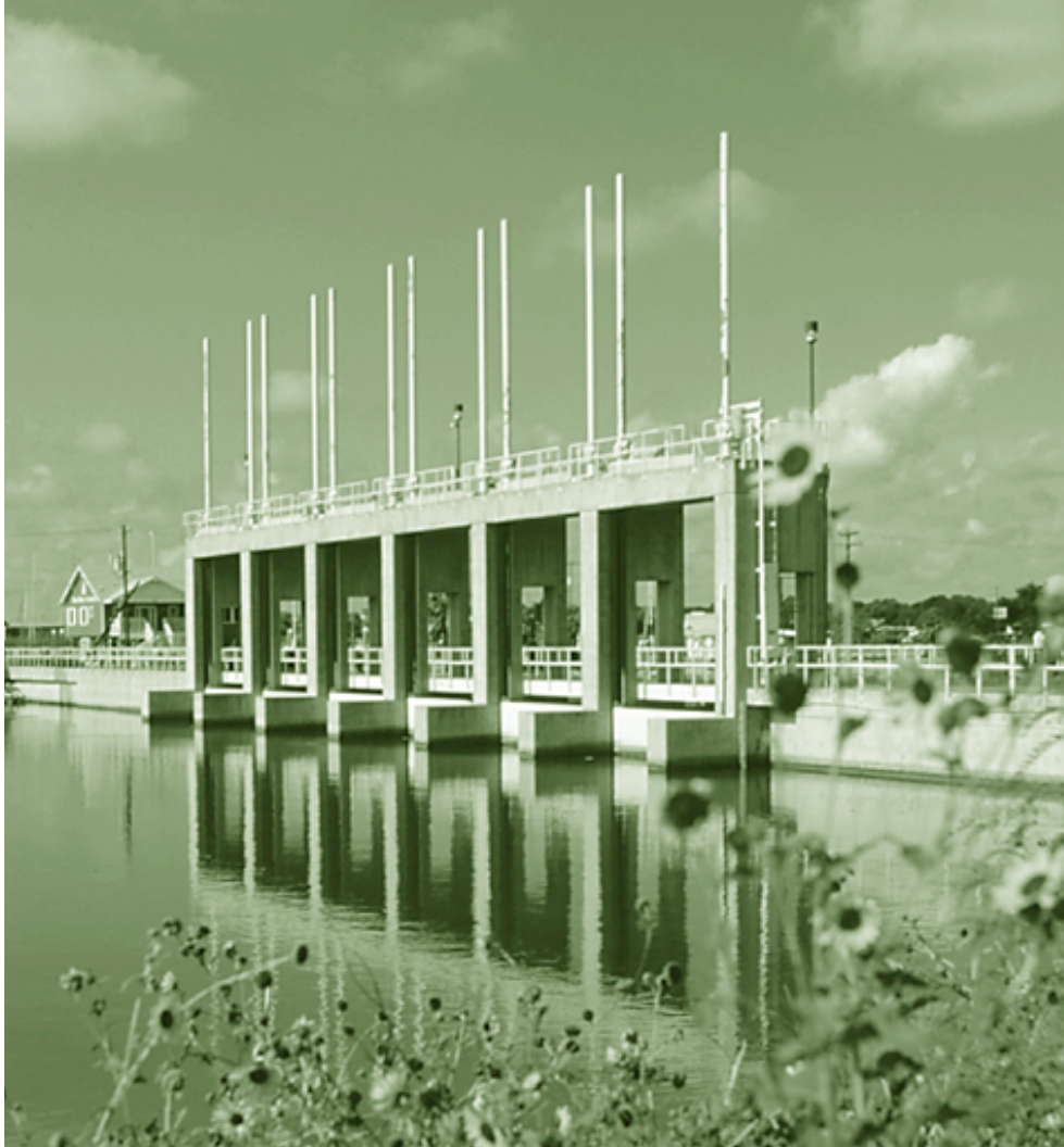
Each of the six, 20'x20' flood gates is driven by a 20 hp electric motor and provided with emergency power generation. The gates are opened when stormwater runoff causes the Clear Lake water level to exceed the Galveston Bay level.
